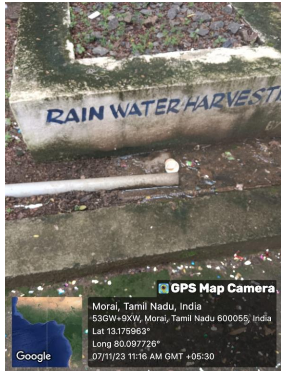
Rainwater Collection System at Block 24
