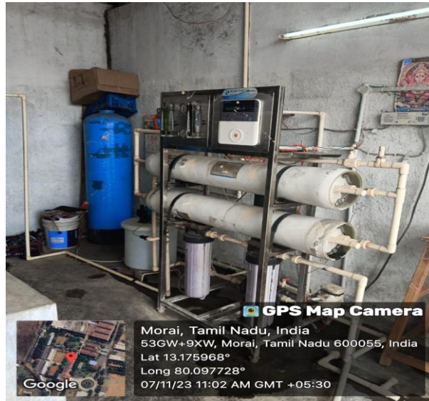
Fig- 5.Reverse Osmosis and Control Unit
