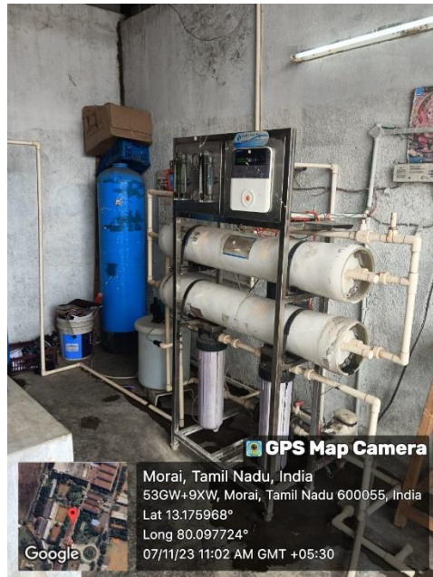
Fig- 3. Reverse Osmosis Plant Including Pressure Sand and Activated Carbon Filter
