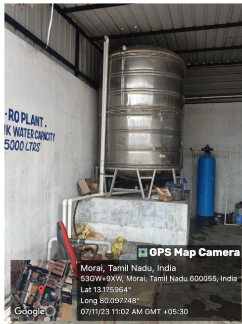
Fig- 4. Stainless Steel Water Collection Tank
