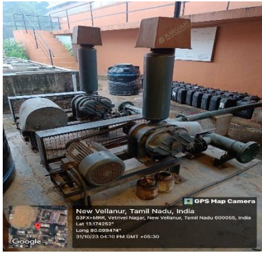
Fig- 1. Pumping and Flow Control House
