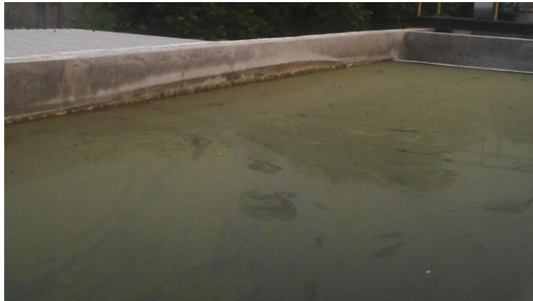
Fig- 10. Settling Tank
