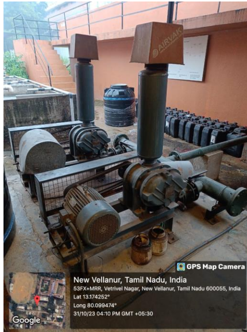
Fig- 12. Blower and Filter
