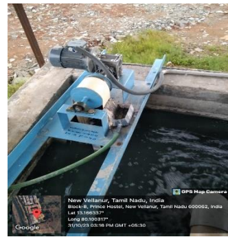
Fig- 4. Aeration Tank and Sedimentation
