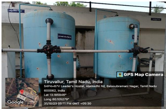
Fig- 3. Sand Filter and Activated Carbon
