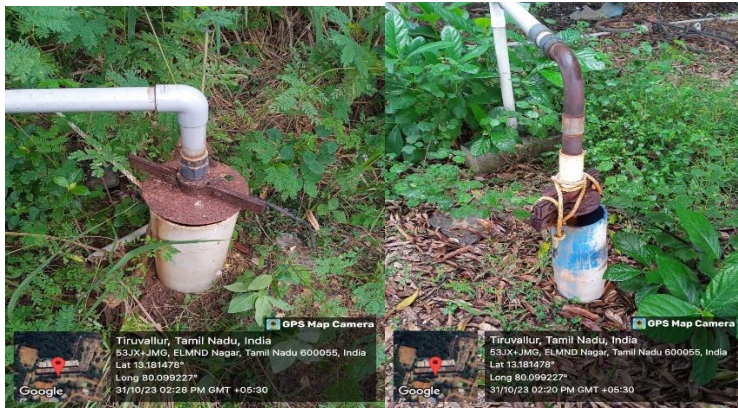
Fig- 3 Aquifers extraction for B-3 Hostels
